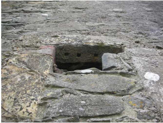
Bar holes blocked window (M)
