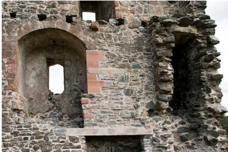
Second floor window (Q)
